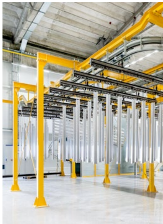
Modern solvent-free powder coating system with low water and energy consumption, pre-treatment tunnel with passivation (corrosion protection), and automated powder application with a recovery system.
